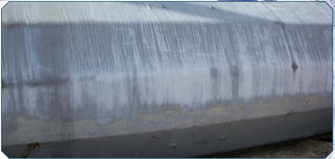
Figure 1: Wet Storage Stain
