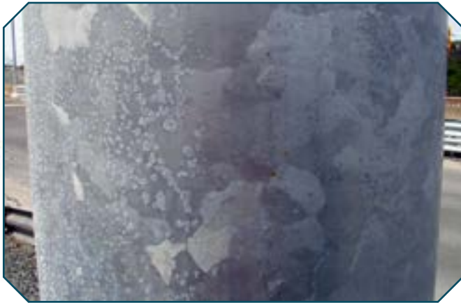
Figure 7: Light wet storage stain
